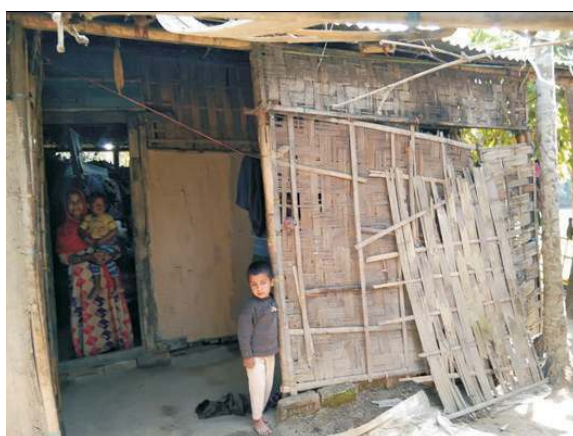
Photograph depicting condition of a shelter of a household from fisherman community, BairagiChawk Part I, Karimganj
