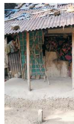
Photograph depicting condition of shelters of shitalpati mat weavers community, Boleswar Part VI village, Karimganj
